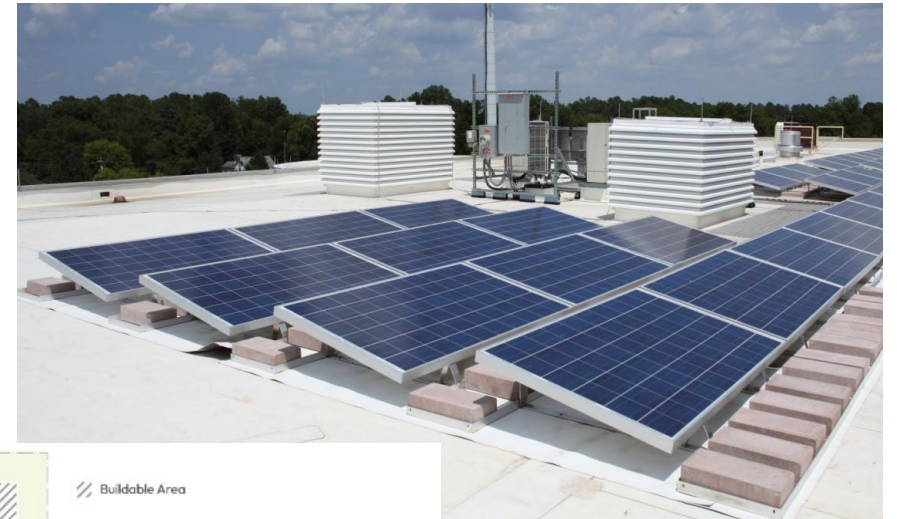
Town Hall rooftop solar
