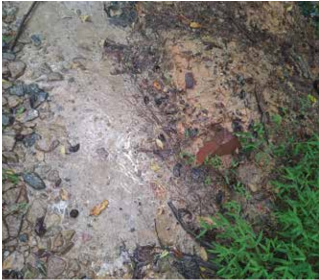
Evidence of site erosion
