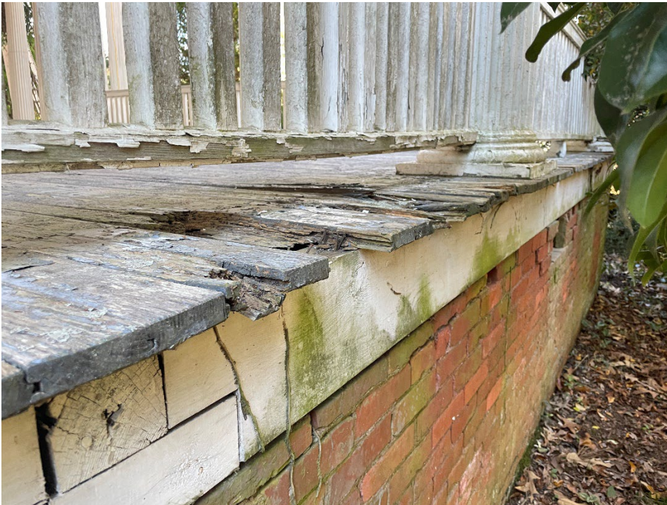
Photo 2: Deteriorated porch decking.
