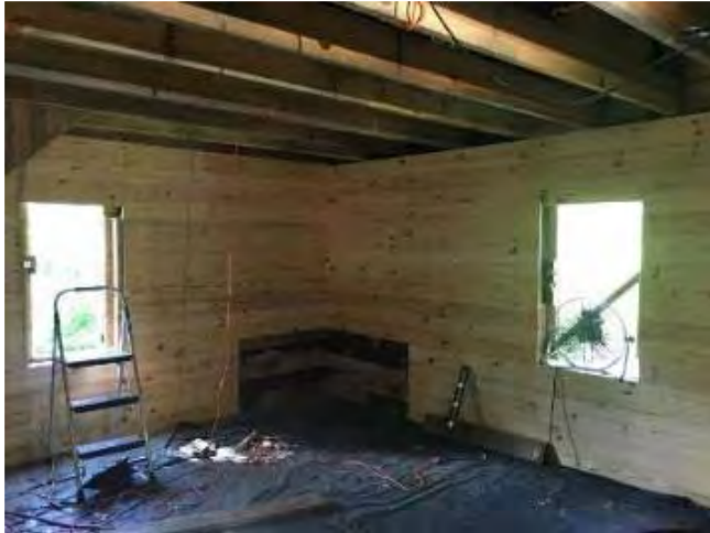
View of the interior of the west side of Ailey Young House after rehabilitation showing the northwest corner. Note a small amount of original wall material was kept for documentation purposes.
