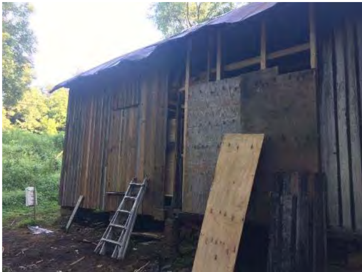
View of the Ailey Young House prior to interior rehabilitation. Note the new board-and-batten siding where the plywood used to be.
