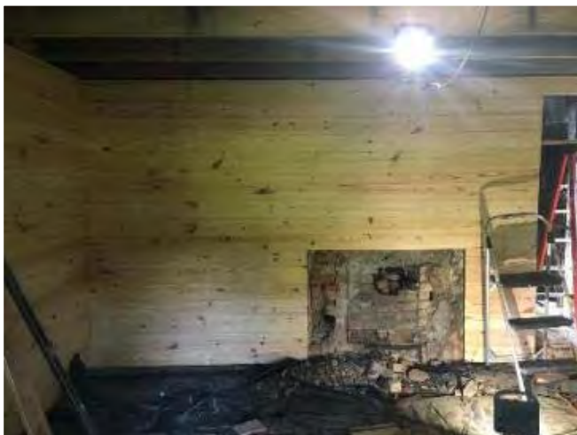
View of the interior of the west side of Ailey Young House after rehabilitation showing the east wall and fireplace opening.
