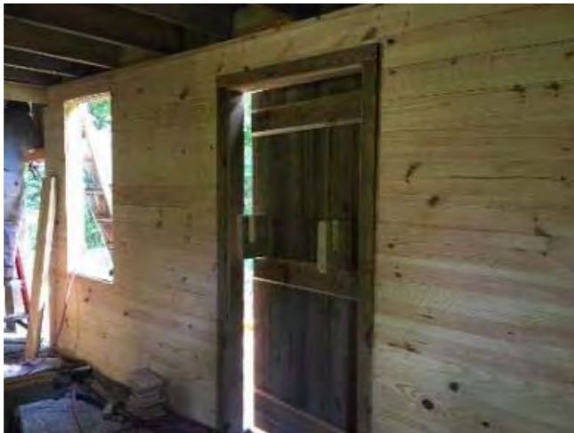
View of the interior of the west after rehabilitation showing the south wall and new door.
