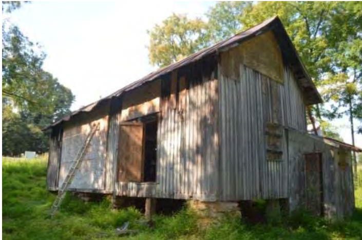
View of the Ailey Young House prior to interior rehabilitation. Note the plywood over the wall next to the ladder.
