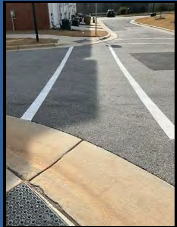
Location: Oakbrook Pass Way; Running Slope GT 12%
