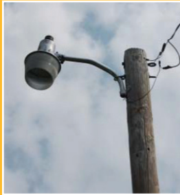
Open Air Security Light on Wood Pole (A33, A81) residential only
